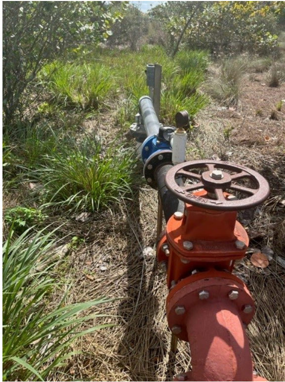
Irrigation - Recharge Well - Hole 11
