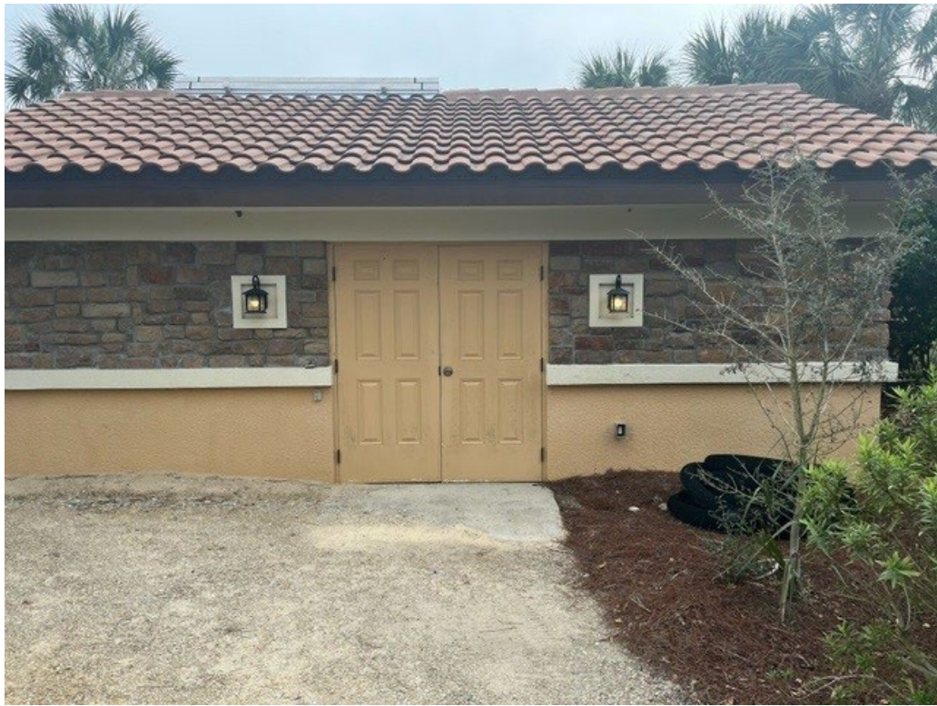
Irrigation - Pump House (External)
