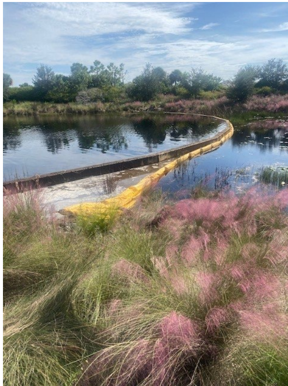
SWM - Flow Way Weir (South)
